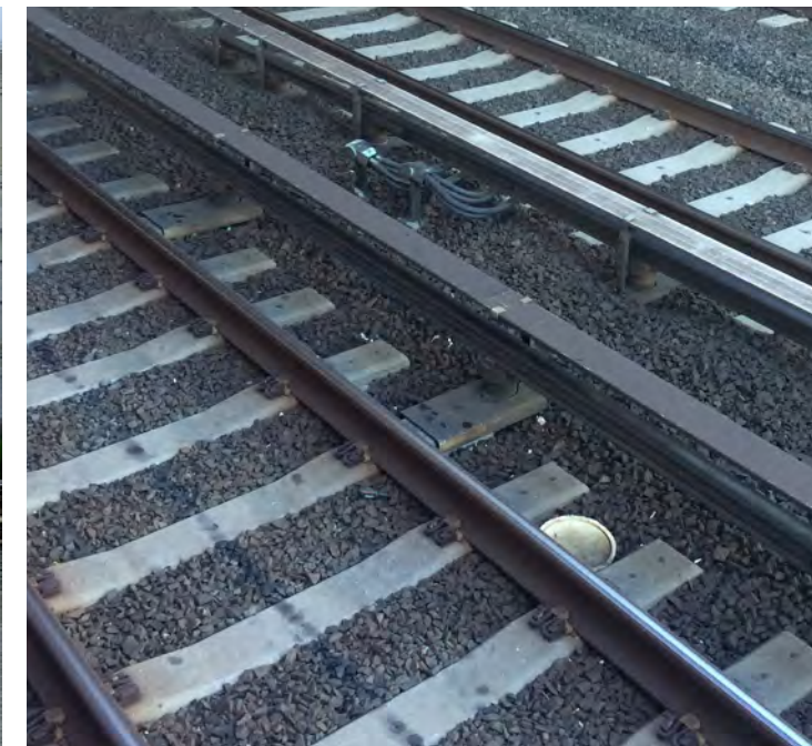
FIGURE 3.4: THIRD RAIL WITHIN SUNNYSIDE YARD
