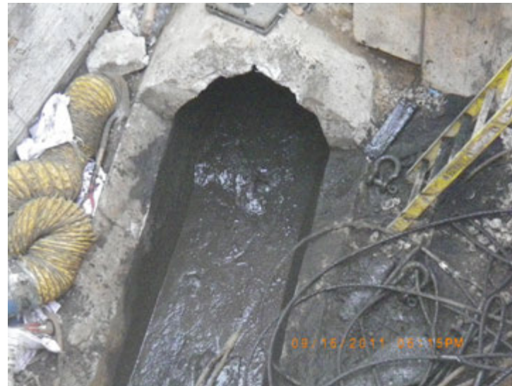
FIGURE D-2 SEWER FULL OF SILT
