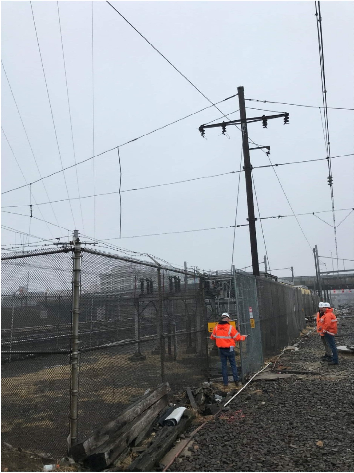
Zone 7 – OCS X Catenary + G02 Substation:
