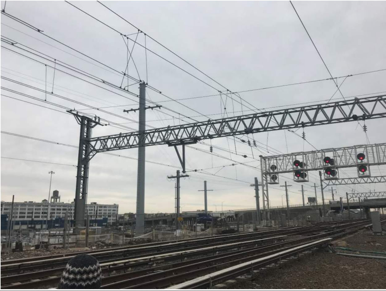
Zone 7 – OCS Truss + Signal Power Monopole + Signal Bridge:
