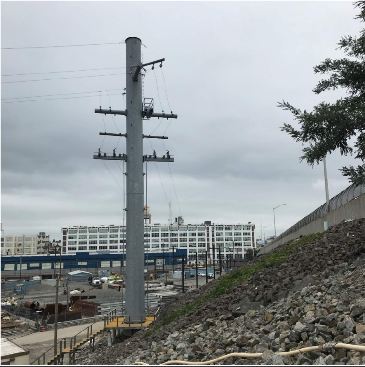
Zone 7 – Signal Power Monopole:
