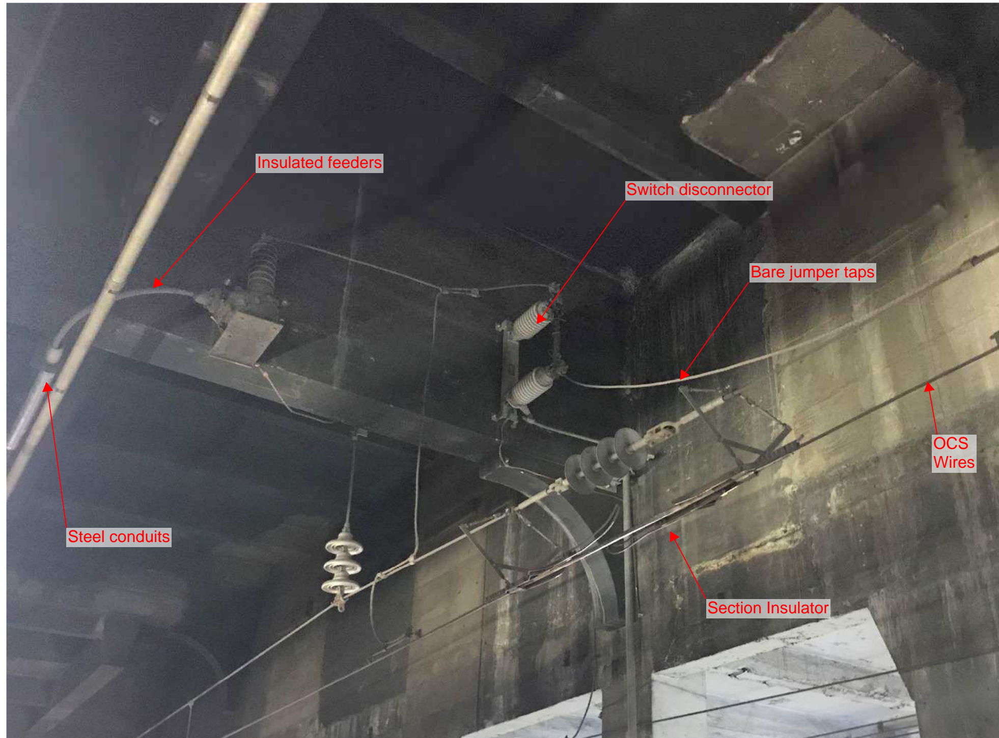
Penn Station - 12kV Sectionalizing
