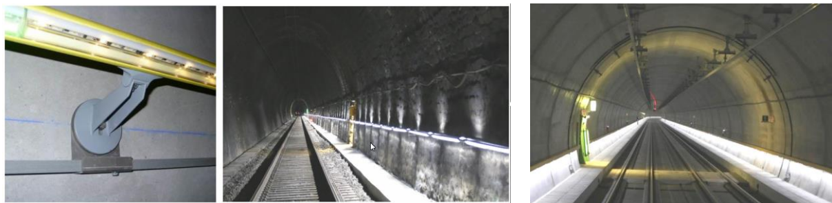
Figure 2.1 - Example for hand rail integrated LED lighting for emergency and maintenance operation
